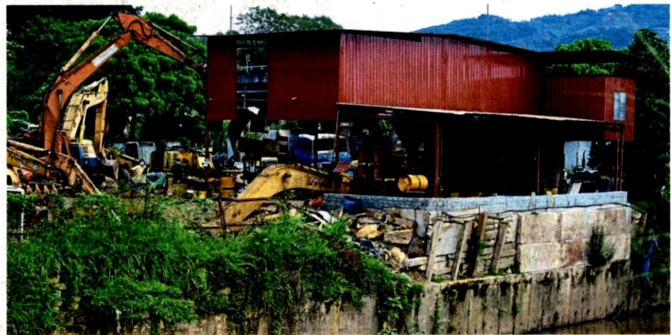
Torn down: MPS enforcement officers demolishing an illegal factory operating along Sungai Rawang in Kampung Dato Lee Kim Sai, Selangor. — SIA HONG KIAU/The Star
